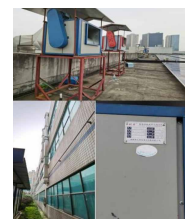
Equipment for centralized collection and treatment of welding fumes
