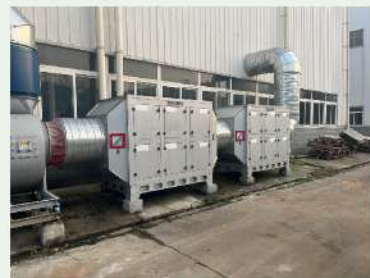
▲ Paint Refinishing Exhaust Gas Treatment Equipment
